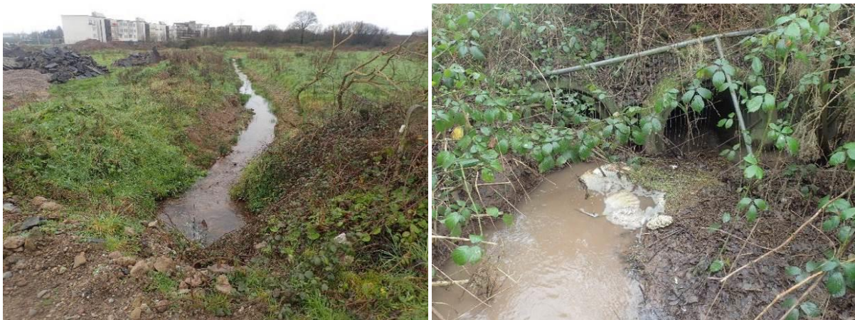
Plate 5.13 Drainage ditch (FW4) that flows south-west through site and exits the site via concrete pipes.
