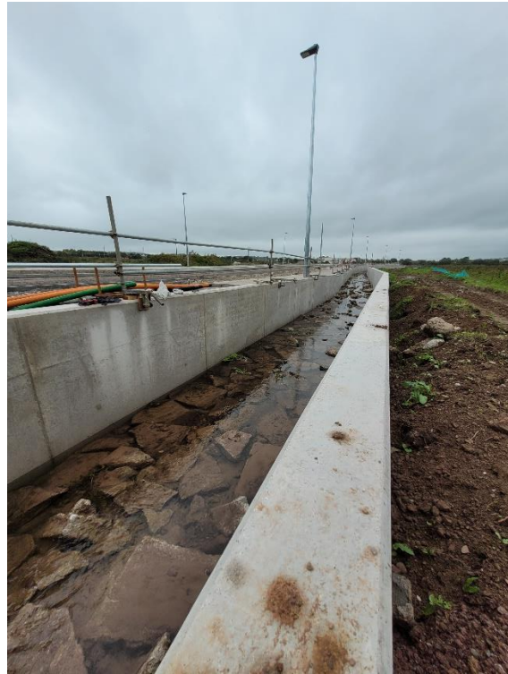
Above right – culverted engineered interceptor channel.
